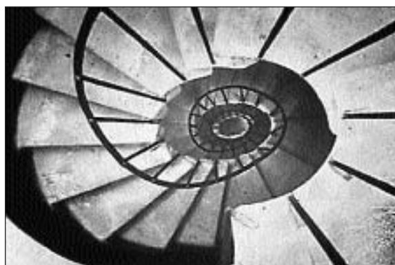
Fig. 6. One of the staircases hidden in the thickness of the corner walls of the central hall.
